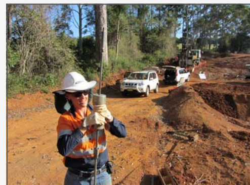
Above: Sarah Marsanich conducts a soil test at the Esk-Hampton Road construction site
