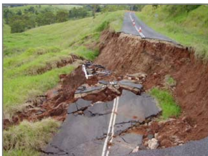
Above: shows extent of land slip damage along Anduramba Range Road looking north.
