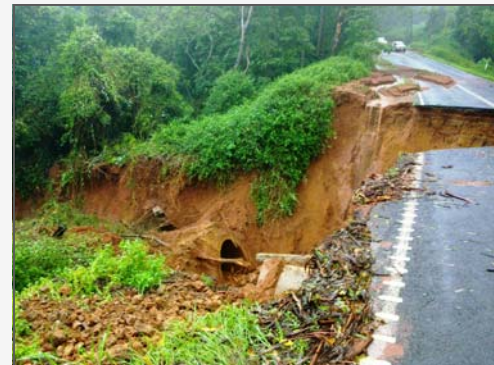
Above: Esk-Hampton Road showing the collapsed culvert immediately after the flood in January 2011
