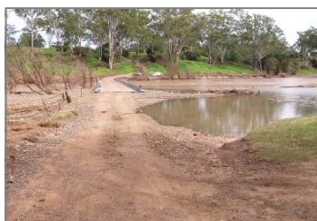
Above: showing damage to Banks Creek Road.
