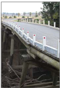
Above: damage to Stokes Bridge
