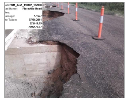
Above: damage on a section of Floraville Road.
