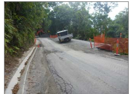
Above showing damage
