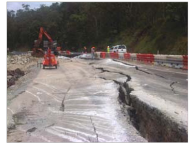
Above: Damage at Claytons Gully, Cunningham Highway
