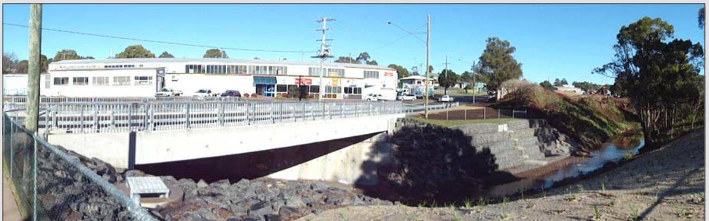
Above: The opening of Jellicoe Street bridge represents a major reconstruction milestone for Toowoomba residents
