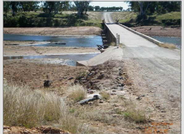
Above: scouring at the Cloncurry River Bridge Approach
