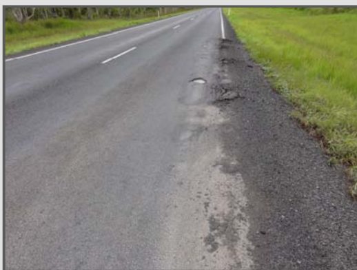
Left: 2011 Post-Natural disaster Damage to pavement and shoulder evident on 9 February 2011
