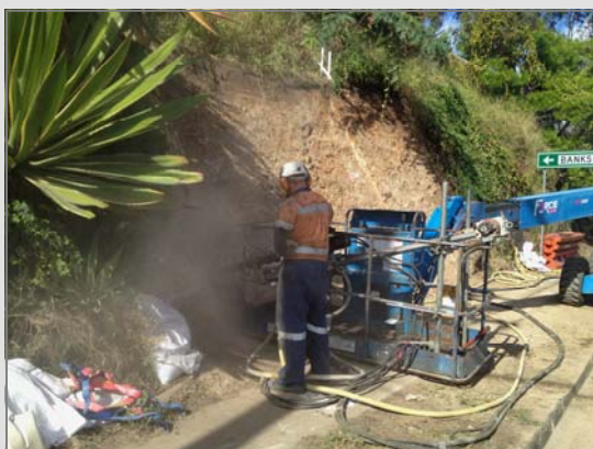
Above: First retaining wall on eastern side of Wardell Street during the works – 31 May 2012
