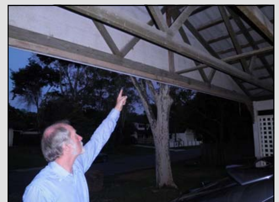
Above: The flood height mark is still visible on the facade
