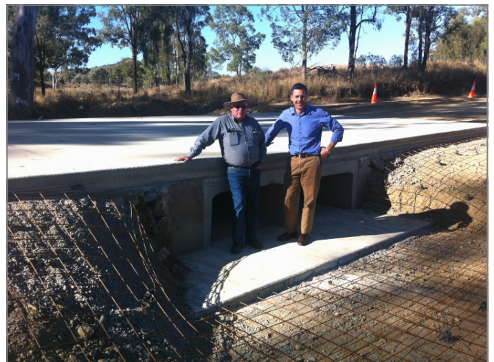
Above: Jim Watson, Works Manager Banana Shire Council and Queensland Reconstruction Authority CEO Graeme Newton inspect reconstruction works at Roys Road. Banana Shire Council's reconstruction works are well progressed, and Council has an overall schedule to complete the works by June 2013.
