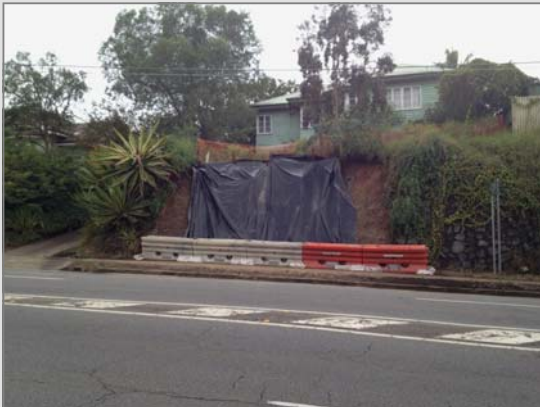
Above: First retaining wall on eastern side of Wardell Street before repair works – 30 May 2012
