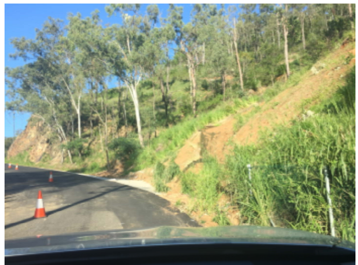
Above: Minor damage to Pilbeam Drive after Severe Tropical Cyclone Debbie
