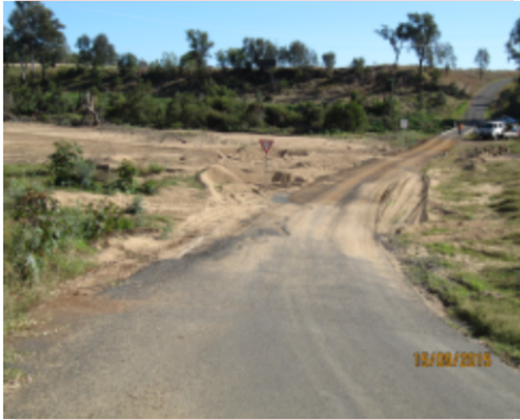
Damage caused by Tropical Cyclone Marcia in 2015
