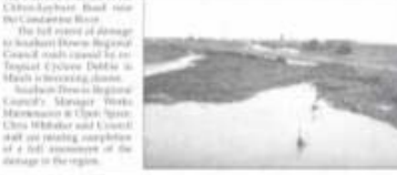
PHOTO: Debris built up under the Kings Creek Bridge following Ex-Tropical Cyclone Debbie.
