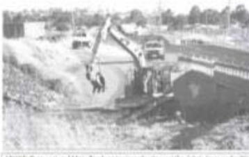
PHOTO: Transport and Main Roads contractors clearing out the debris from under Kings Creek Bridge on Thursday, more than five months after the worst weather system hit the region.
