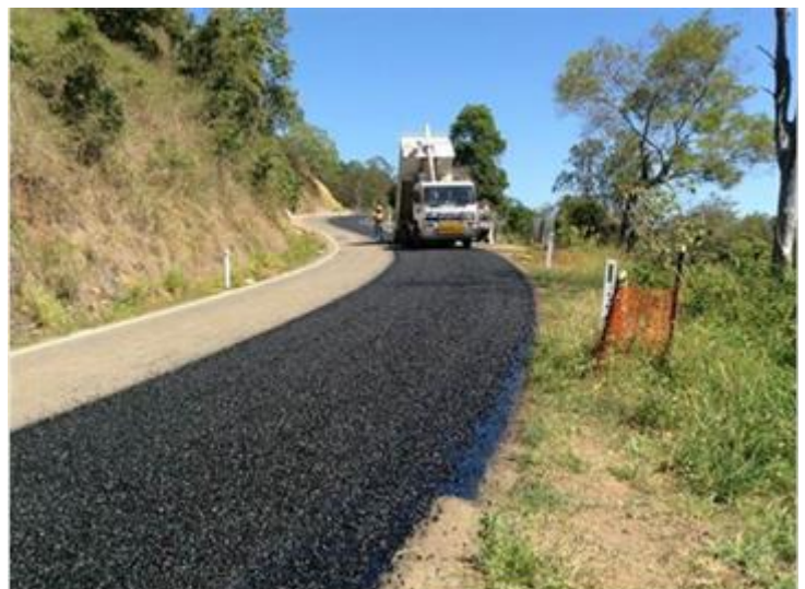
Placement of final seal at a site during the reconstruction of Kenilworth-Brooloo Road
