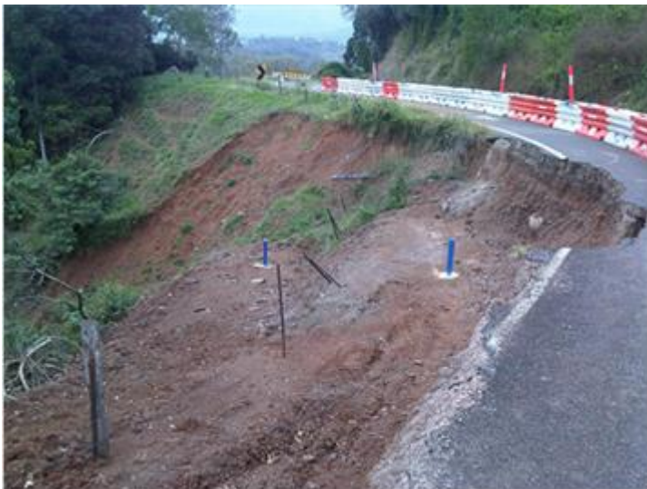
Downhill landslip damage prior to reconstruction works commencing at the main damage location
