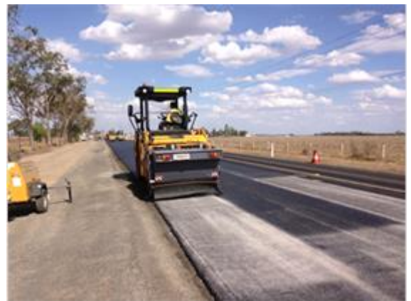
Works underway on Warrego Highway near Dalby – multi-tyre roller with grit spreader for stone mastic asphalt works
