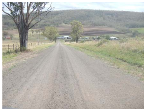
Left: damage (far left) and following reconstruction works (left) to sections of O'Donohue Road
