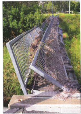
ROBT Debris hangs from the damaged footbridge a year after the event.
