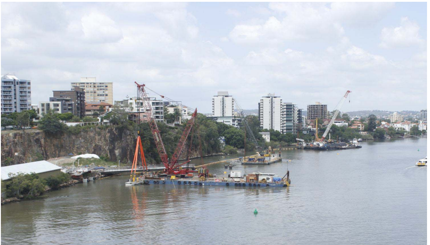
Riverwalk progress, including the installation of the first girder which will form the walkway
