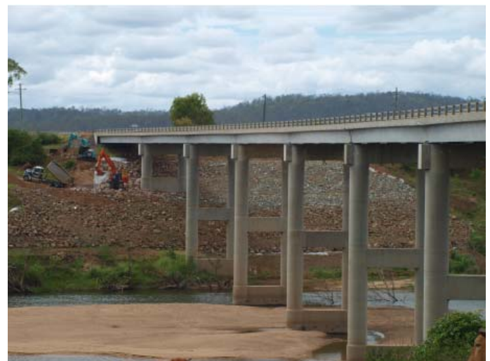
Above: works underway on Tim Fischer Bridge, Bruce Highway to place rock fill and an external boulder armour following embankment slips during the 2013 events
