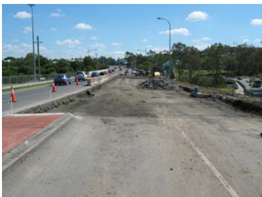
Above: flood damage to One Mile Bridge (top) and the Betterment works underway (bottom)
