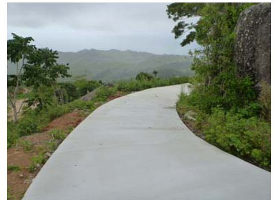
Above: damage to Upper Mount Bentley Road from the 2013 event (top) and the completed Betterment works following Tropical Cyclone Dylan in February 2014 (bottom)
