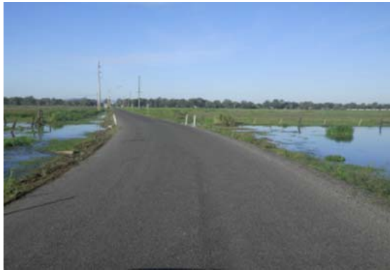
Damage to (top), and following repairs to Fiddes Street, Rockhampton
