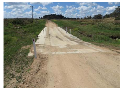
Above: damaged floodway on Gomoran Douglas Road (top) and following restoration (bottom)
