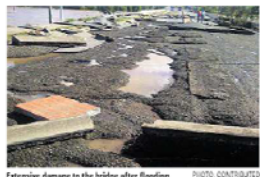
EXTENSIVE damage to the bridge after flooding. PHOTO CONTINUED
