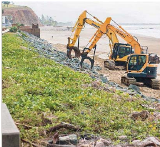
WORKS: JRT excavators repair beachside rock walls at Yeppoon's Main Beach. PHOTO: CONTRIBUTED
