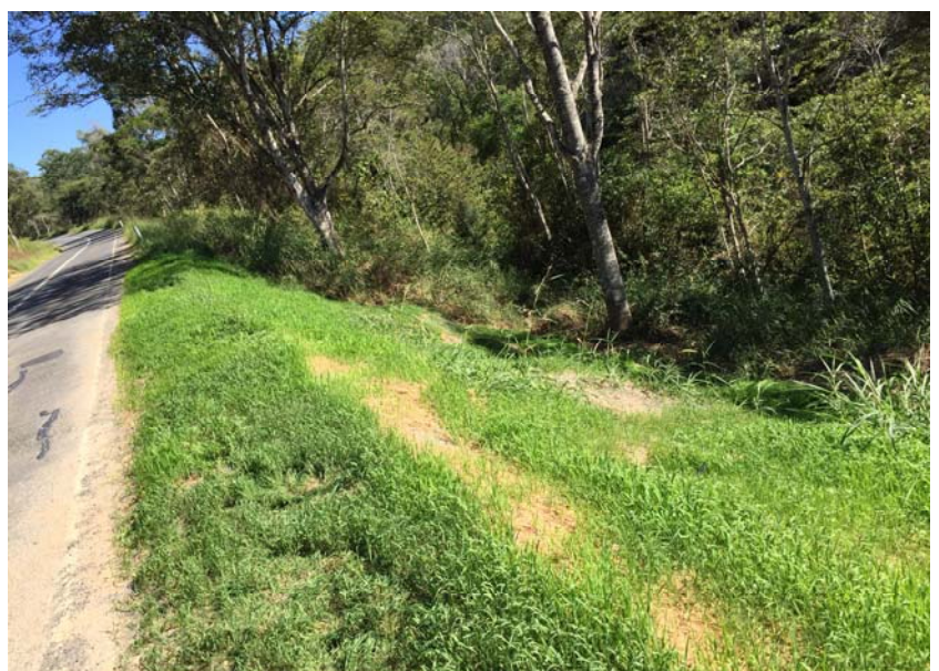
Right: Uphill slope stabilisation and downhill slip repairs completed on Noosa Shire Council's Cooroy Belli Creek Road
