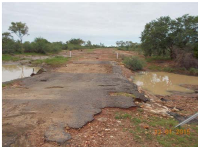
Damage to Gregory Downs–Camooweal Road from Western Queensland Heavy Rainfall and Flooding (January 2015)
