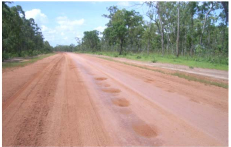
Weipa-Mapoon Road before Betterment funding when the unsealed road was susceptible to damage
