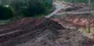
Deep Creek Bridge, Gayndah-Mundubbera Road under construction. Council acknowledges the Natural Disaster Relief and Recovery Arrangements (NDRRA) funding is a joint Commonwealth and State Government program.
