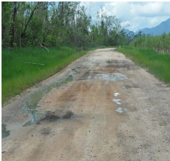
Above: Old Cardwell Road - damage following Cyclone Yasi
