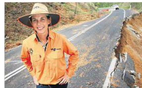
REPAIRS: Roadtek's Kirsty Hinchliffe on the Mount Morgan range. PHOTO: CHRIS ISON ROK12013ROAD7
