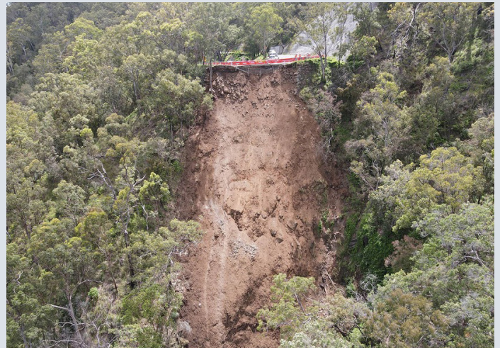
Lamington National Park Road – major landslide site (December 2021)
