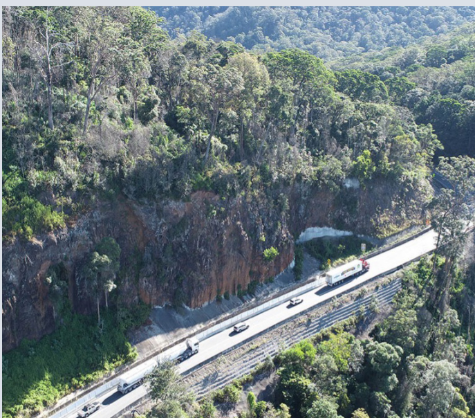
Cunninghams Gap damage site
