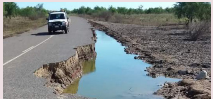
Wills Developmental Road (Julia Creek–Burketown) – damage from Northern and Central Queensland Monsoon and Flooding (March 2023)
