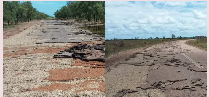
Wills Developmental Road (Julia Creek–Burketown) – pavement delamination and scouring as a result of Northern and Central Queensland Monsoon and Flooding (March 2023)
