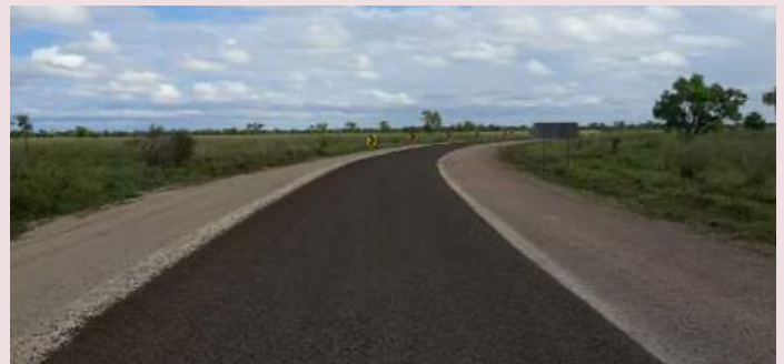
Wills Developmental Road (Julia Creek–Burketown) – pavement delamination and scouring as a result of Northern and Central Queensland Monsoon and Flooding (March 2023)
