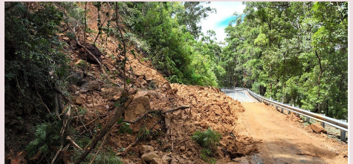
Gold Coast–Springbrook Road – Site 8 landslide following SEQ Rainfall and Flooding event (February 2022)
