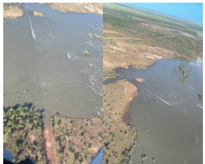
Aerial view of flood-impacted road access in Burke Shire Council
