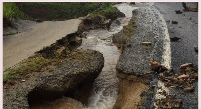
Mackay–Eungella Road – shoulder scour (January 2023)
