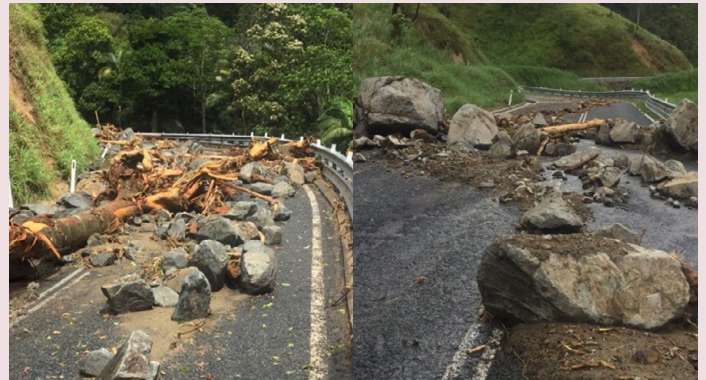
Mackay–Eungella Road – landslide site (January 2023)
