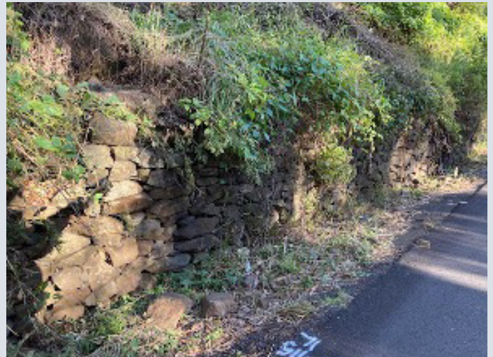
Tamborine Mountain Road – damaged dry-stone wall (March 2021)
